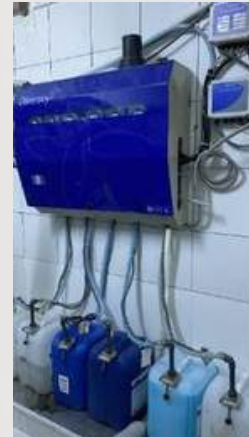
Laundry Dosing System
